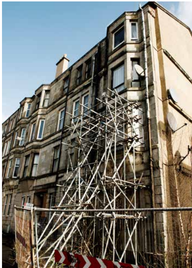
Awaiting improvement, flats in Orchard Street, Paisley
